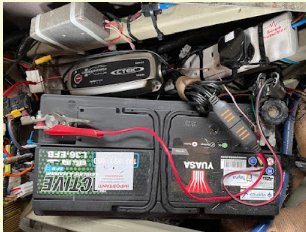
The battery charger just goes in here when it's needed. It is also used for car and motor cycle batteries.
